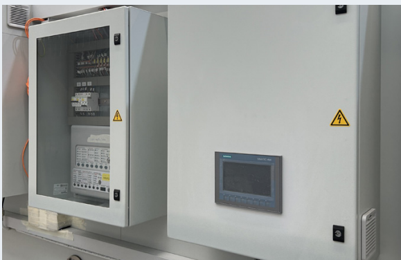
SAFETY CONTROL SYSTEMS PLC
