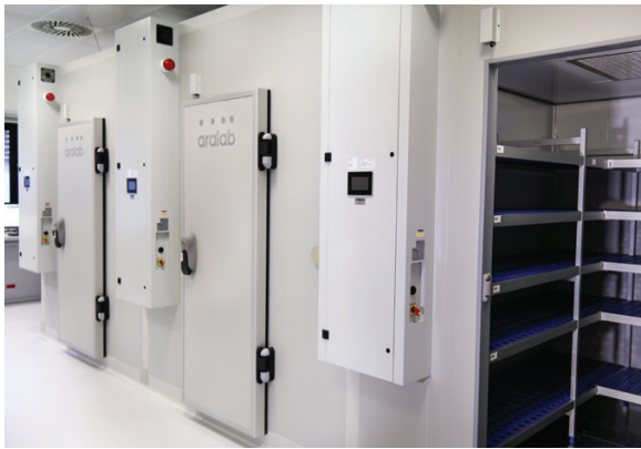
STABILITY ROOMS TURNKEY PROJECT BY ARALAB
