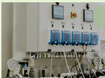
Hydroponic Irrigation (pH and EC control)
